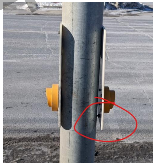
Figure 9: Loose push button on east side pole
