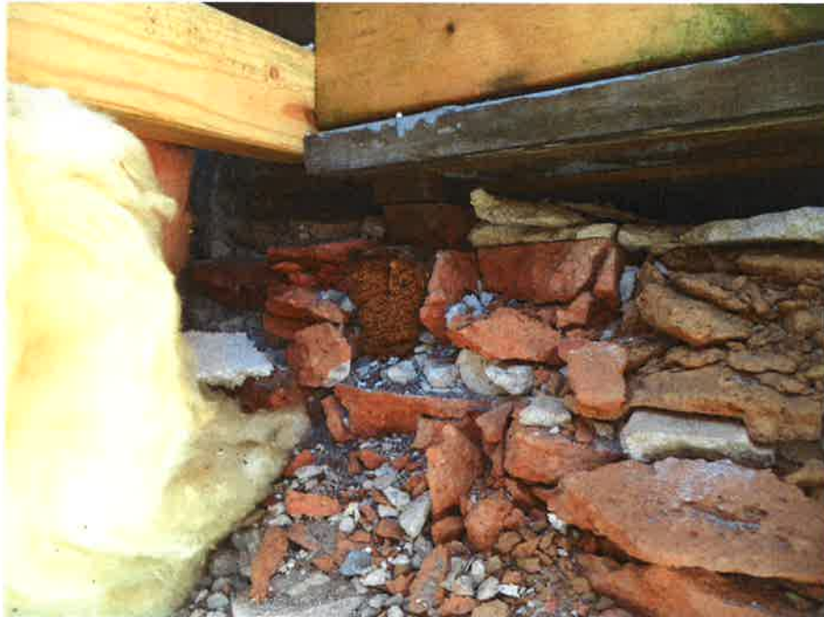
6 Close-up view of deteriorated clay brick infill below former ground floor window
