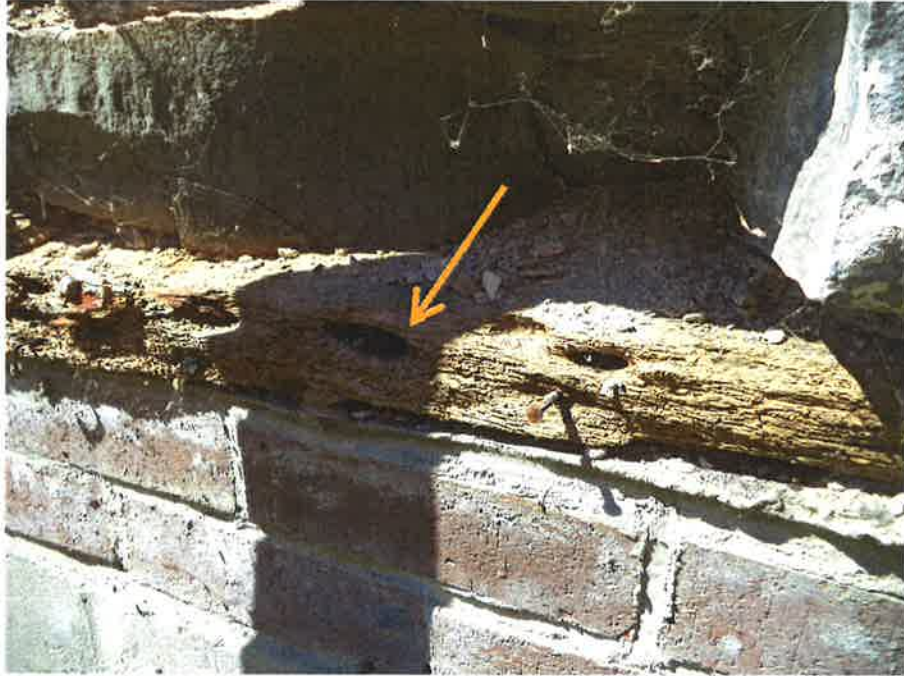
5 Close-up view of decayed wood lintel
