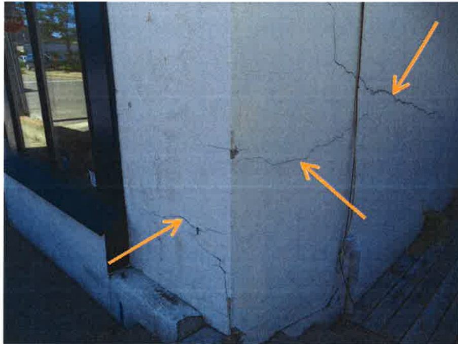
10 Showing miscellaneous cracking in stucco at NW corner
