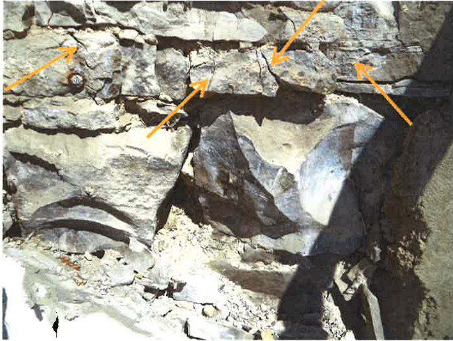
9 Close-up view showing numerous fractures in stone units and poor mortar condition
